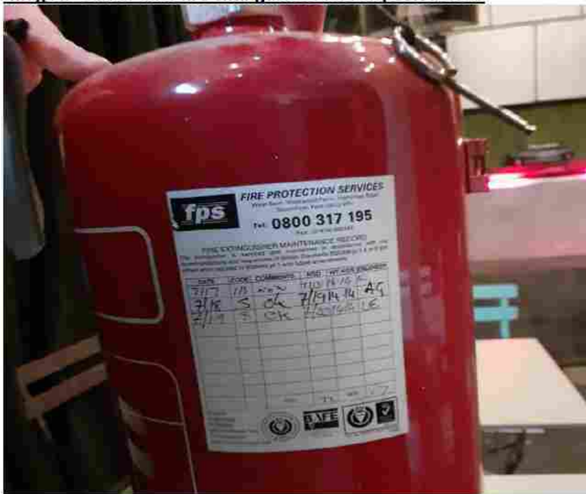
Image 2 -Out of date fire extinguishers last inspected 2019
