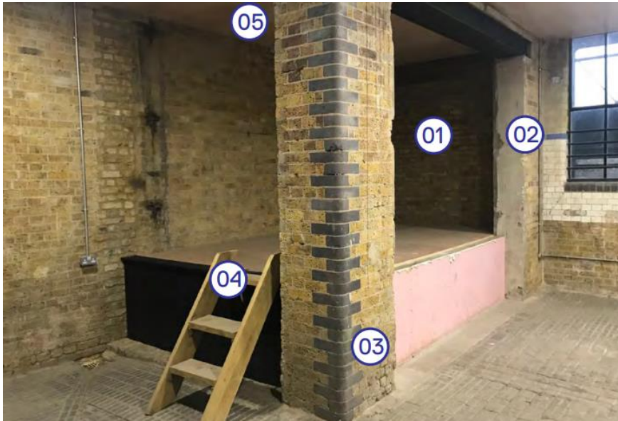
Figure 10: Interior view of first floor looking west, with pier to be demolished labelled as '3'
