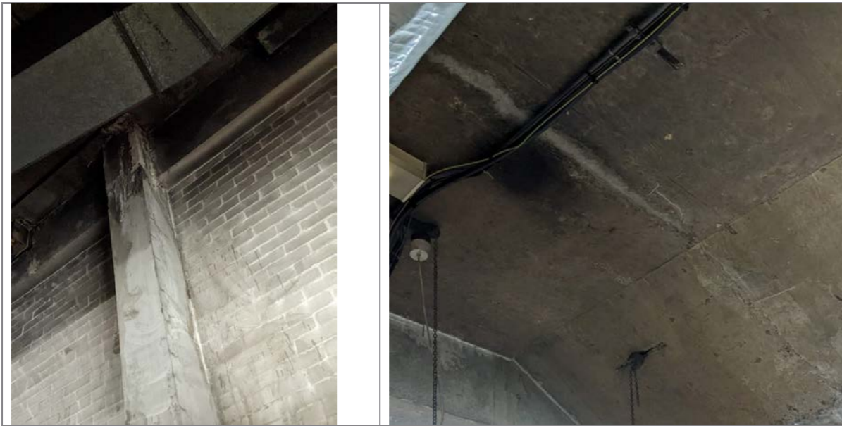
Figure 4 - example of previous, poorly repaired concrete column, basement level
