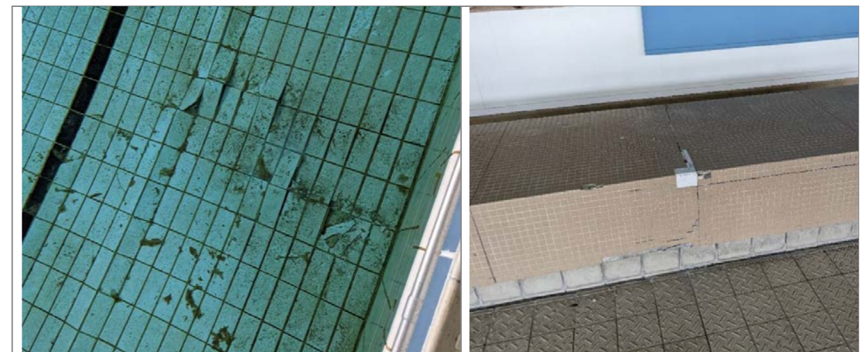
Figure 7 - main pool base tiles cracked/ lifted. Pool base requires local concrete repair with new membrane.
