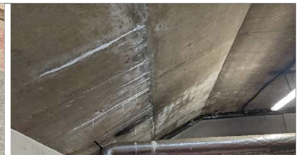
Figure 3 - seepage through concrete pool box at construction joints requiring treatment
