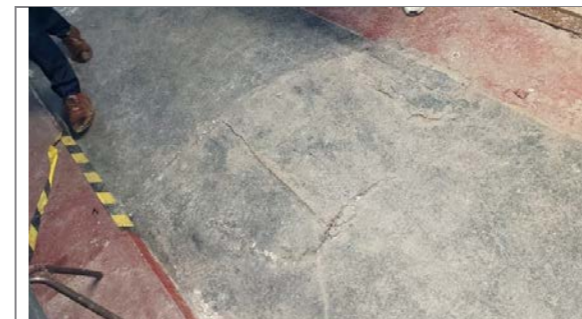
Figure 2 - locally damaged sections of basement floor slab requiring break-out and reinstatement
