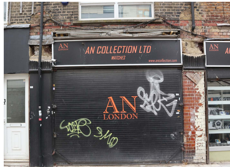
Nos.5-7 Leyden Street Inconsistent drainage layout - in front of corbel on the left and behind on the right
