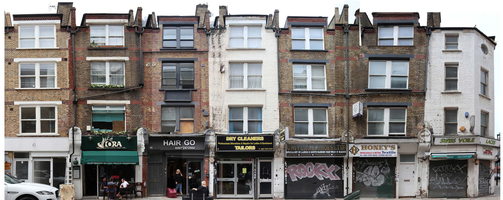
Nos.7-19 Wentworth Street Existing condition of facade drainage
