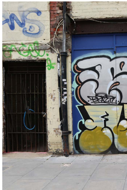
No.1 Leyden Street Rainwater pipe from building above drains into large foul pipe
