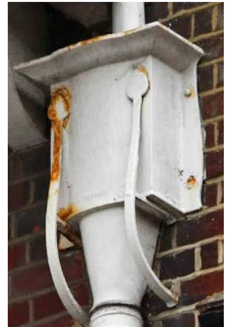
Decorative bespoke fixing brackets to rainwater hopper
