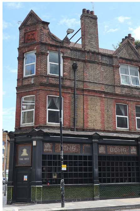
The Bell PH Downpipe draining behind shopfront
