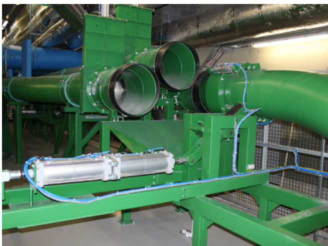
Fig. 13. Collection pipes associated with an Automated Waste Collection System. Image courtesy of Envac.
