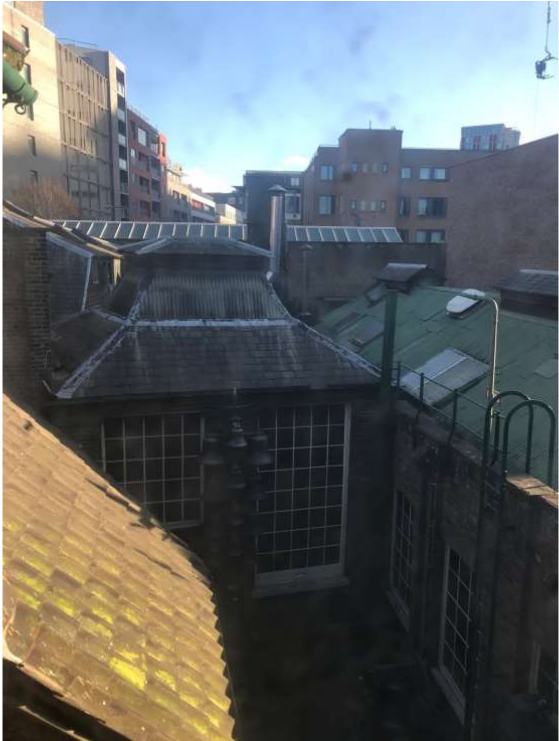
View from upper floors of foundry (facing south towards 1980s extension and Mulberry Street)
