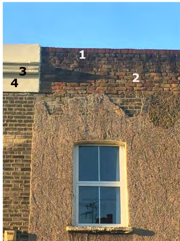
Cement coatings and lack of mortar can reduce the life of the brickwork
