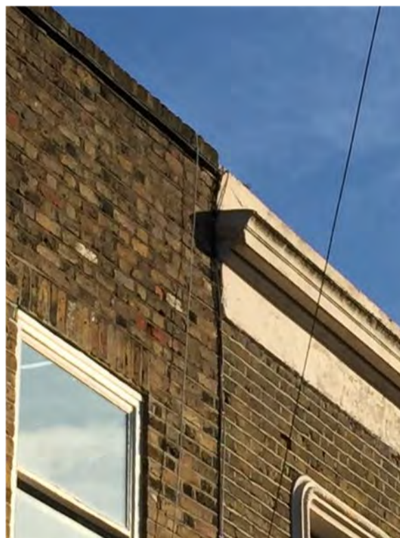
All render requires regular maintenance and redecoration; cracks lead to decay
