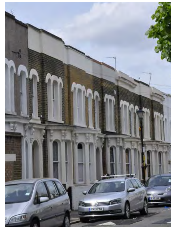
Loss of cornices reduces the architectural character
