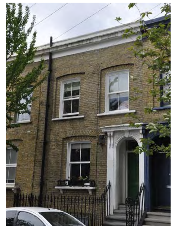
Driffield Road cornice penetrated by pipework
