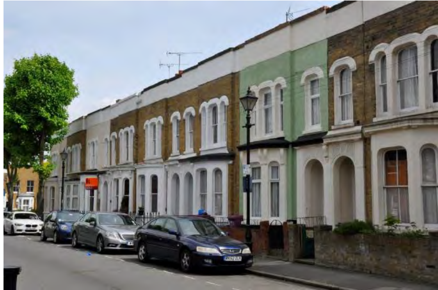
Antill Road. This photograph shows the alternating recess to the front elevations, some of which have been painted, and all in this image are missing their original cornices.
